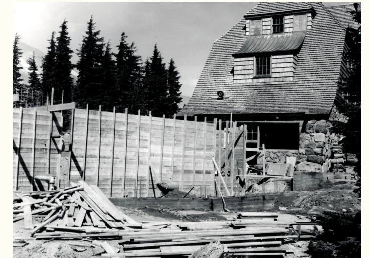
Construction of the Lodge swimming pool was on its way in August 1958".
