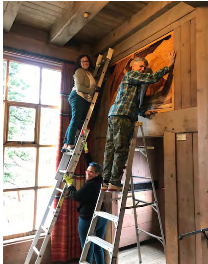
Nina Olsson and helpers reinstall the lobby wood marquetry after it received its conservation treatment.
